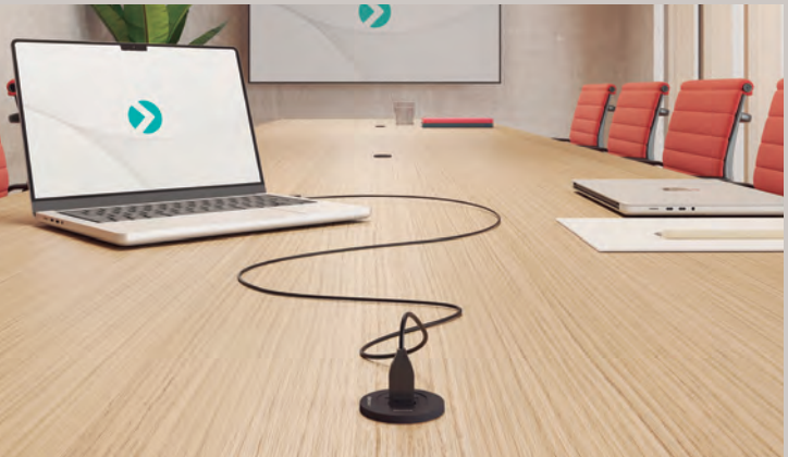
Bit Multimedia con conectores HDMI instalados en mesa de reuniones. Bit Multimedia with HDMI connector installed on a meeting table.
